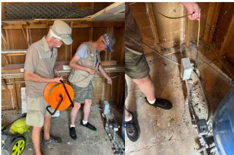
PWOA volunteers Ralph Goff, left, and Budd Watkins test static water level in a well. Photo credit - Matthew Burg
